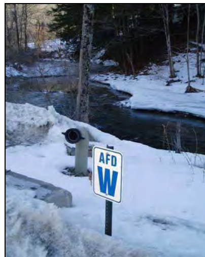
Figure 22: Green River dry hydrant.
