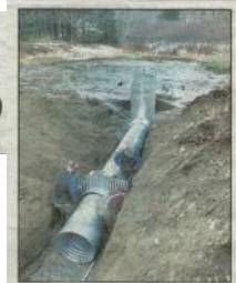
Repairs recently were made to the dry hydrant on Snow Brook Lane in Wells.
